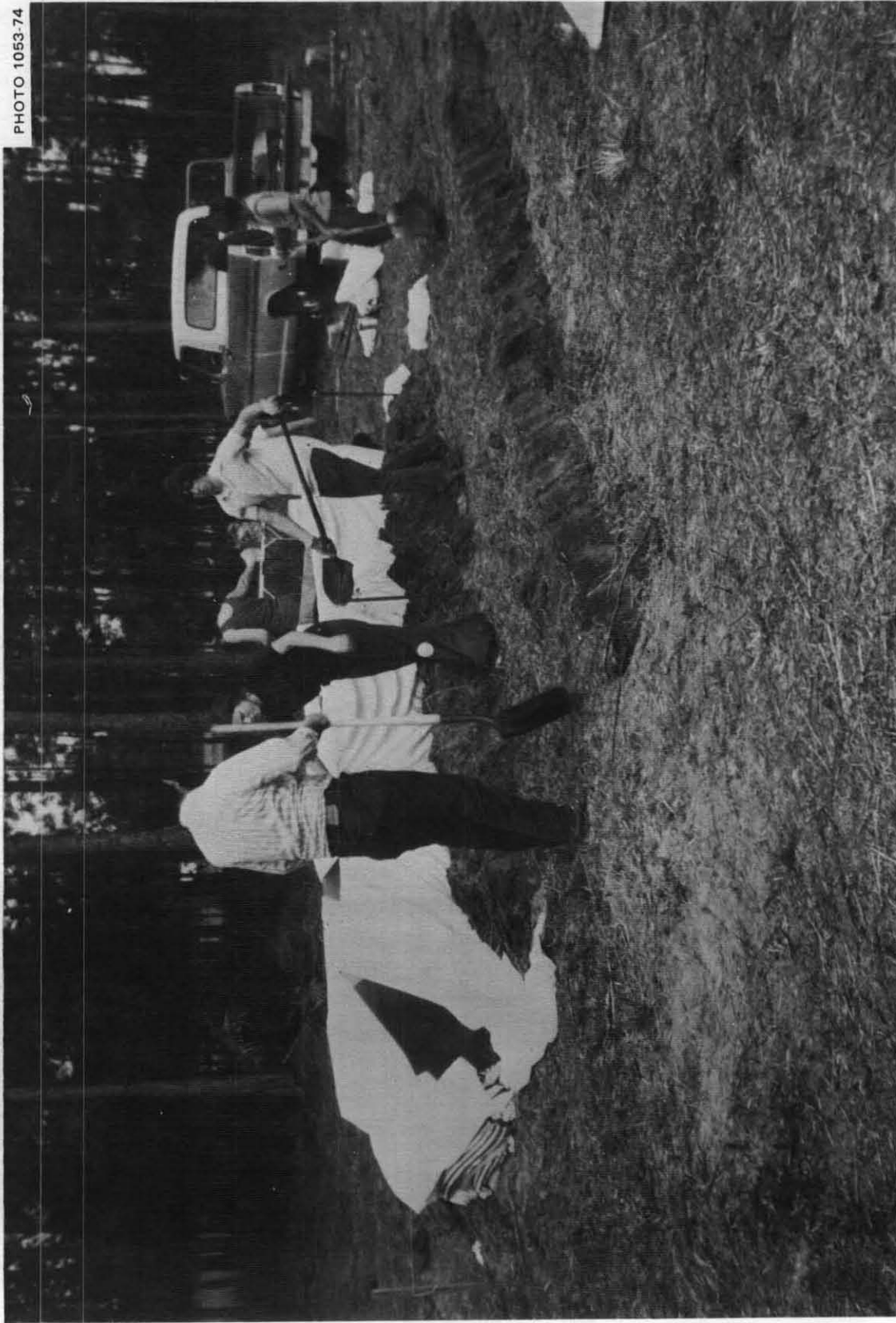
Fig. 5.4. Starting to make the first roll by shoveling earth onto bed sheets that had been placed with 2 ft of their long sides on the ground, with the rest of the sheets temporarily draped over the doors used as forms. This sandy earth could be dug quite easily with shovels.
